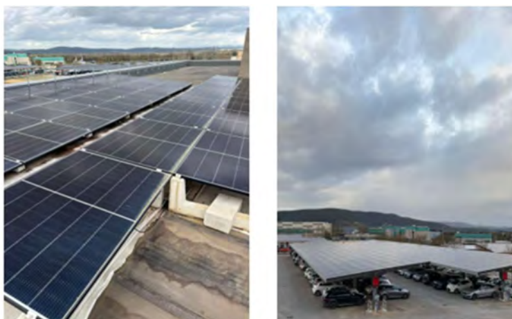
Figure 17 – On the left, a 30 kW photovoltaic system; on the right, a 380 kW photovoltaic system
