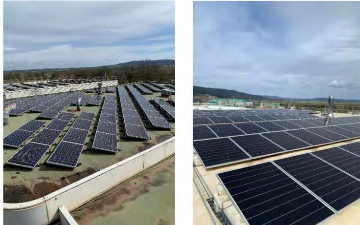
Figure 16 – On the left, a 40 kW photovoltaic system; on the right, a 70 kW photovoltaic system
